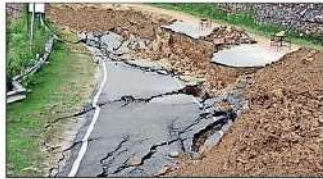
Subsidence on Badrinath highway between Pursari and Malkhan
